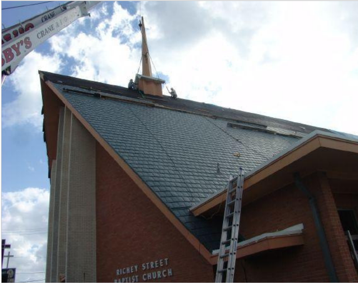
Construction workers dismantle the steeple at Richey Baptist Church to make way for the new one. The church suffered substantial damages after Hurricane Ike. The process with insurance agents has been slow but the church continues to rebuild.
